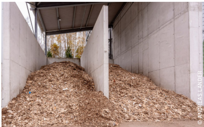
Exemplary fuel storage with regional biomass.
