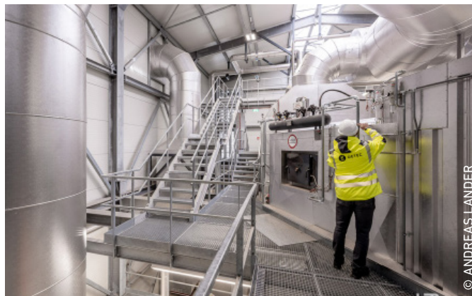
Exemplary boiler house of a biomass heating plant.
